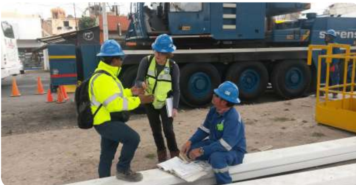
Listening to the crane operator if he understood and uses the best practices is key in an audit process - (internal audit - Mexico on the Toluca project).
