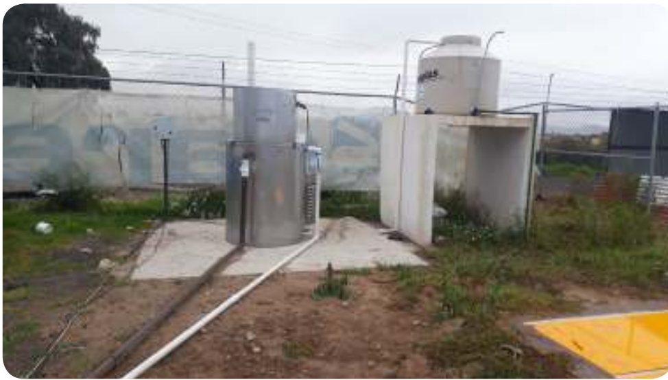
sewage water treatment plant on the yard in Mexico
